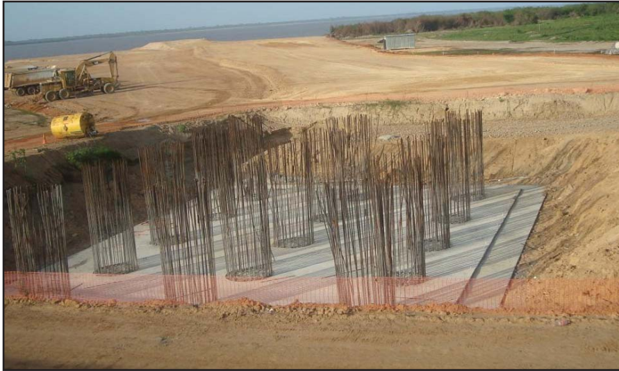
Construction of the foundations was a very difficult logistical challenge, considering that 90% of the foundations are under water half of the year.
